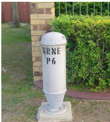
Example of Telstra Pillar.
